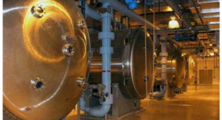
Figure 5. Ozone generators at Carroll Plant.
