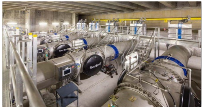
Figure 6. Ultraviolet disinfection units at Carroll Plant.
