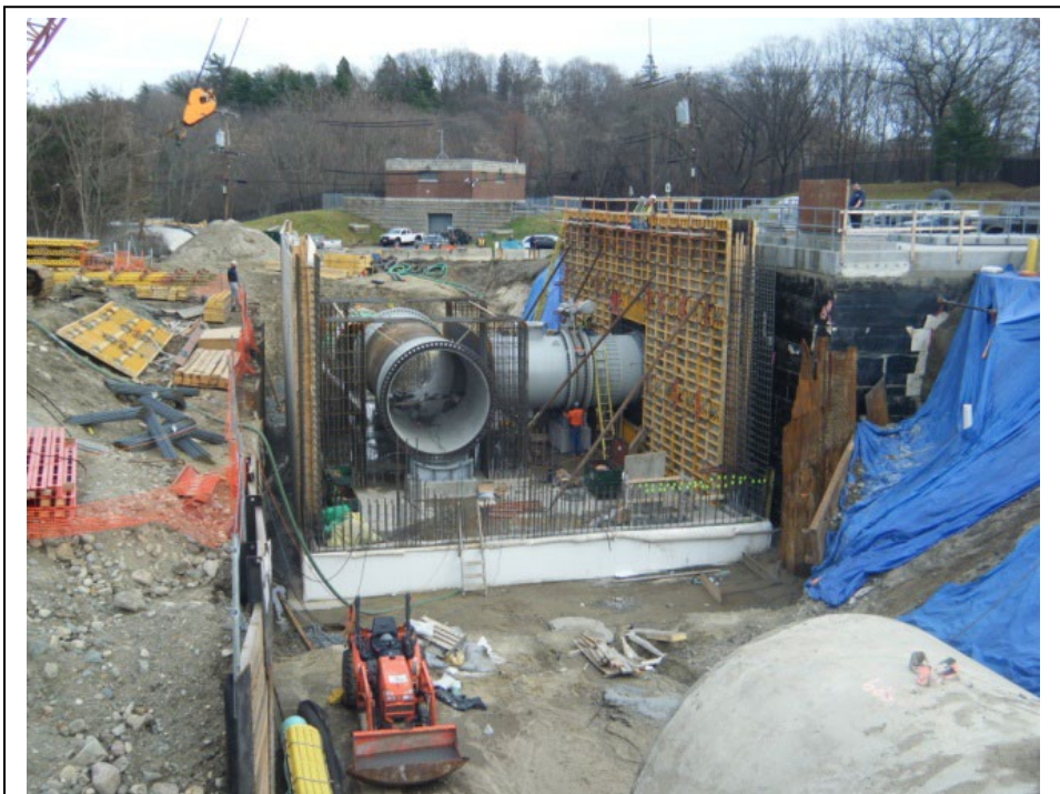
Figure 4. Valve chamber at Shaft 5 connecting MetroWest Tunnel and Hultman Aqueduct (MWRA).
