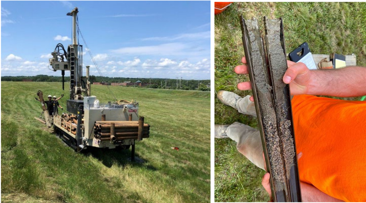
Figure 14. Borings for piezometer installations at North Dike (L), subsurface data collection (R)
