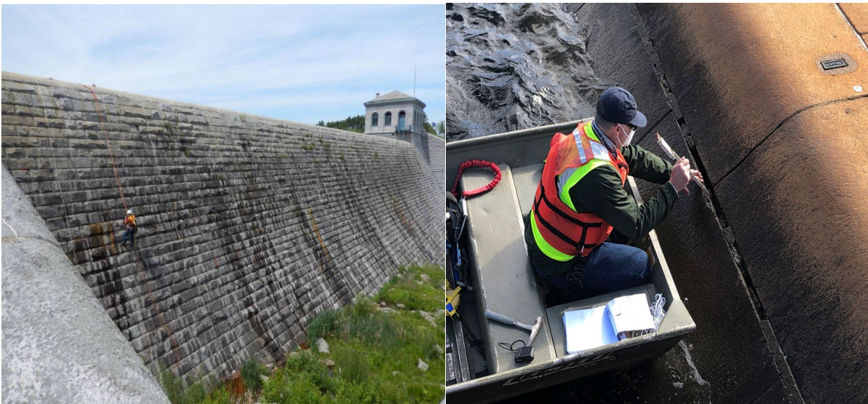
Figure 13. Current condition of Sudbury Dam Spillway downstream face (L) and upstream crest (R)
