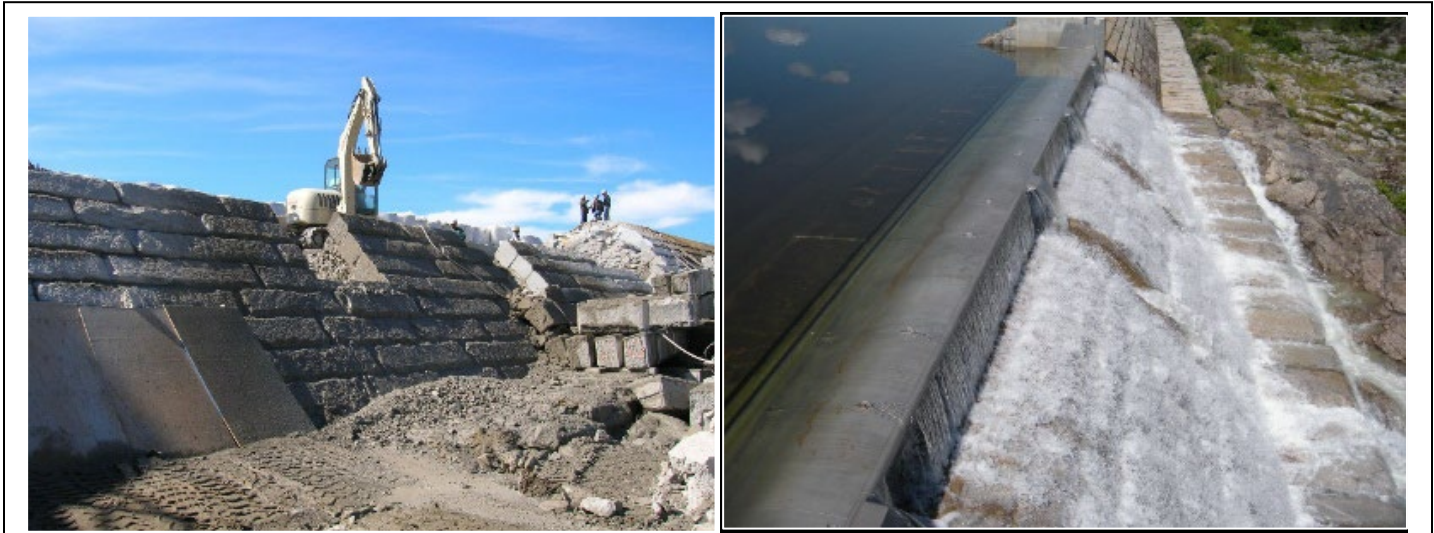
Figure 8. Lower Wachusett Dam spillway (L) to accept new 100-foot-long Crest Gate (R)
