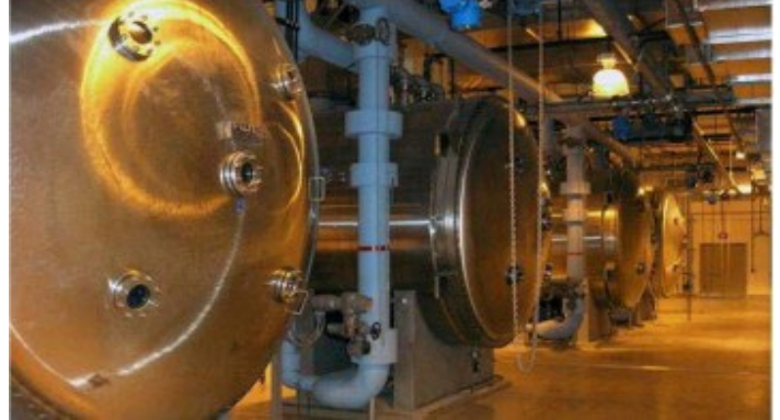
Figure 5. Ozone generators at Carroll Plant.
