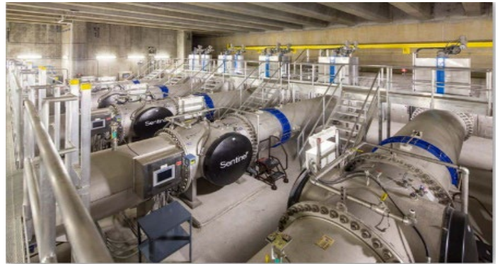
Figure 6. Ultraviolet disinfection units at Carroll Plant.
