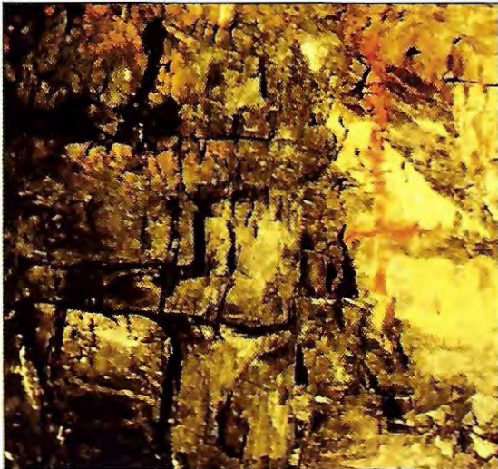
FIGURE 3-47. North-trending diabase dike with columnar jointing and with fault gouge along its border at the Wellesley Extension Intercept Tunnel in Dedham.
