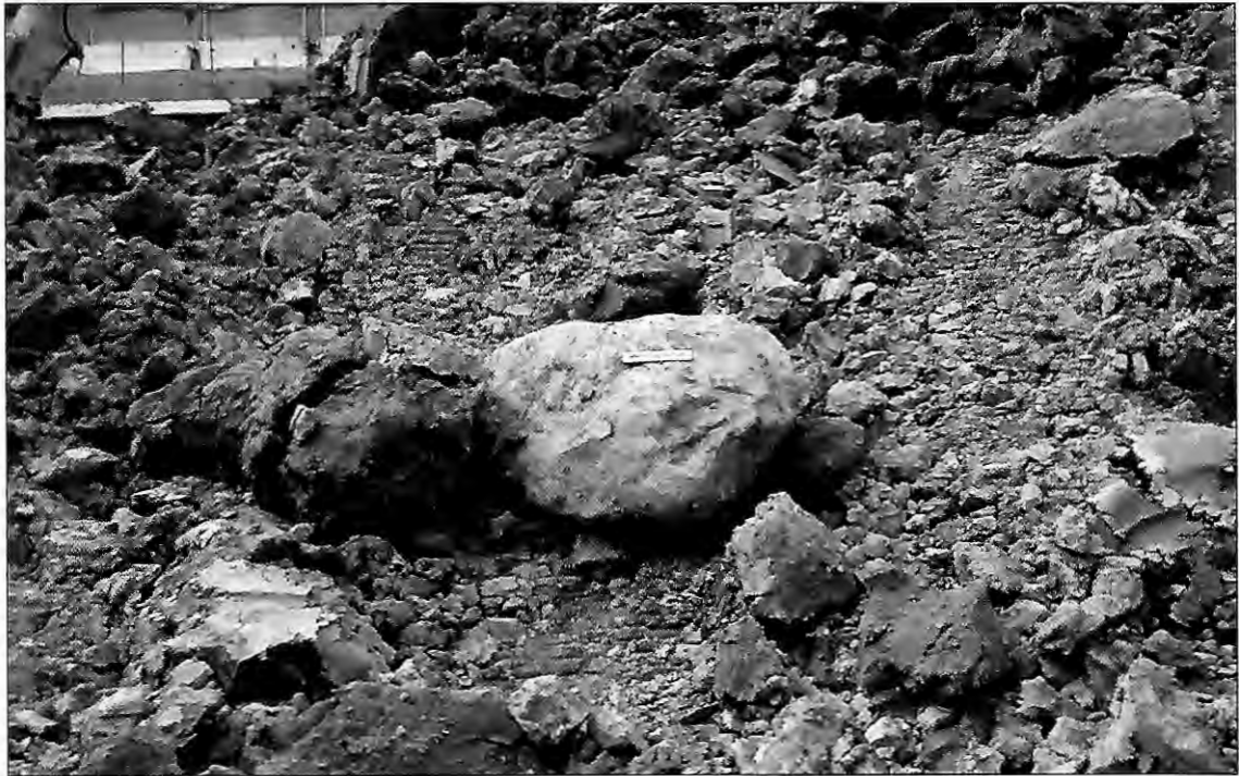
FIGURE 3-97. Marine clay rubble in excavation, including large boulders. (Photo courtesy of Bradford Miller.)
