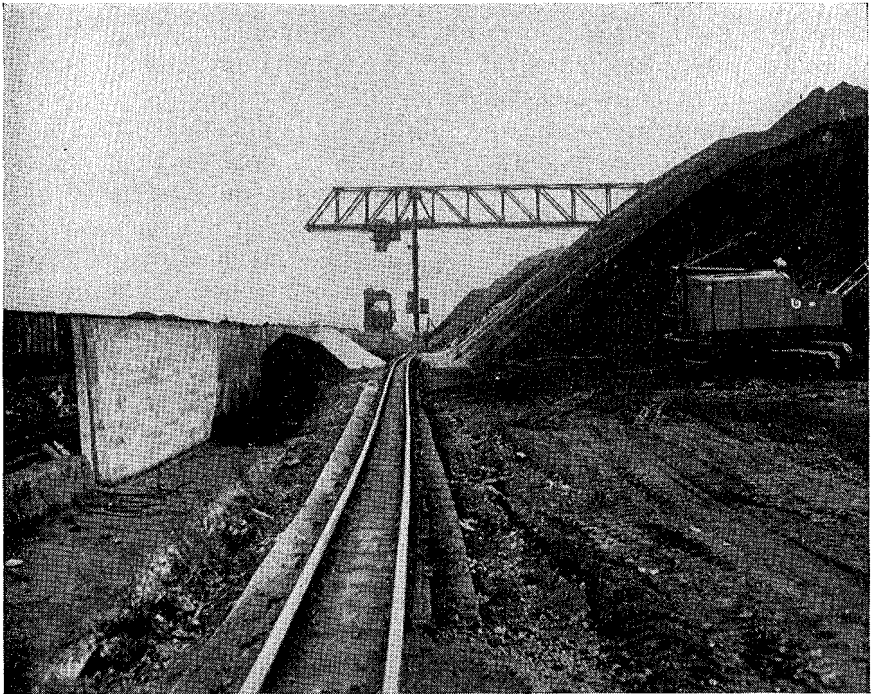
FIGURE 3.—DISPLACEMENT OF ORE BRIDGE TRACK BY HEAVE AND LATERAL MOVEMENT.
