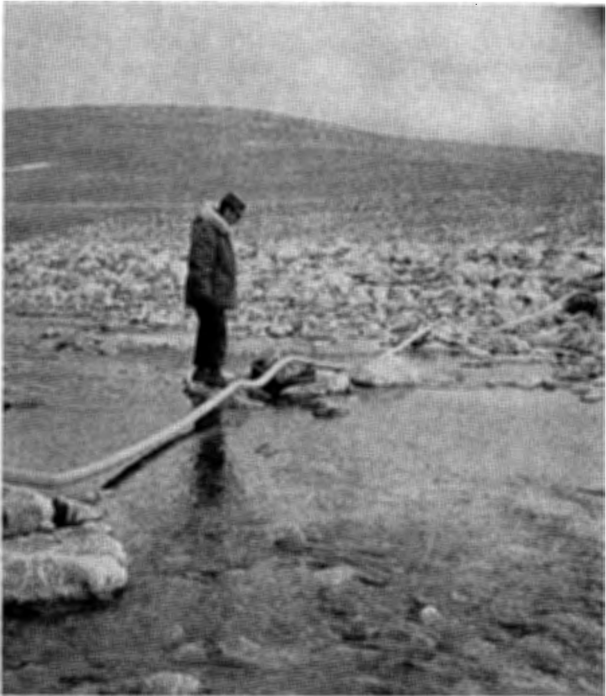
FIGURE 3.—PIPE-LINE DAMAGED BY CONSOLIDATION OF SNOW.
