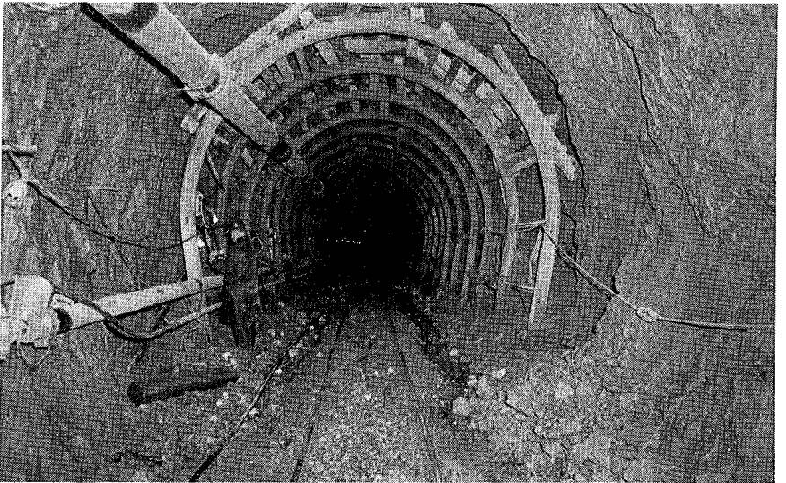
FIG. 10.—LOOKING SOUTHERLY TOWARD LONG SECTION OF STRUCTURAL STEEL, NORTHERN END OF WHICH IS AT STATION 33 + 17. ROCK IS TUFF-BRECCIA OF LYNN VOLCANICS
