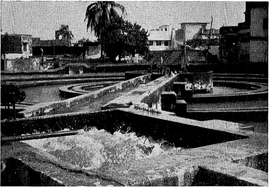
FIG. 5.—MIXING AND FLOCCULATION BASIN AT OLD DACCA TREATMENT PLANT
