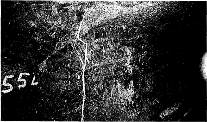
Fig. 15. — Station 280 + 71. Looking east. Red sandstone interbedded with conglomerate. Bedding strikes parallel to tunnel and dips about 25^{\circ} N. 1/19/49.
