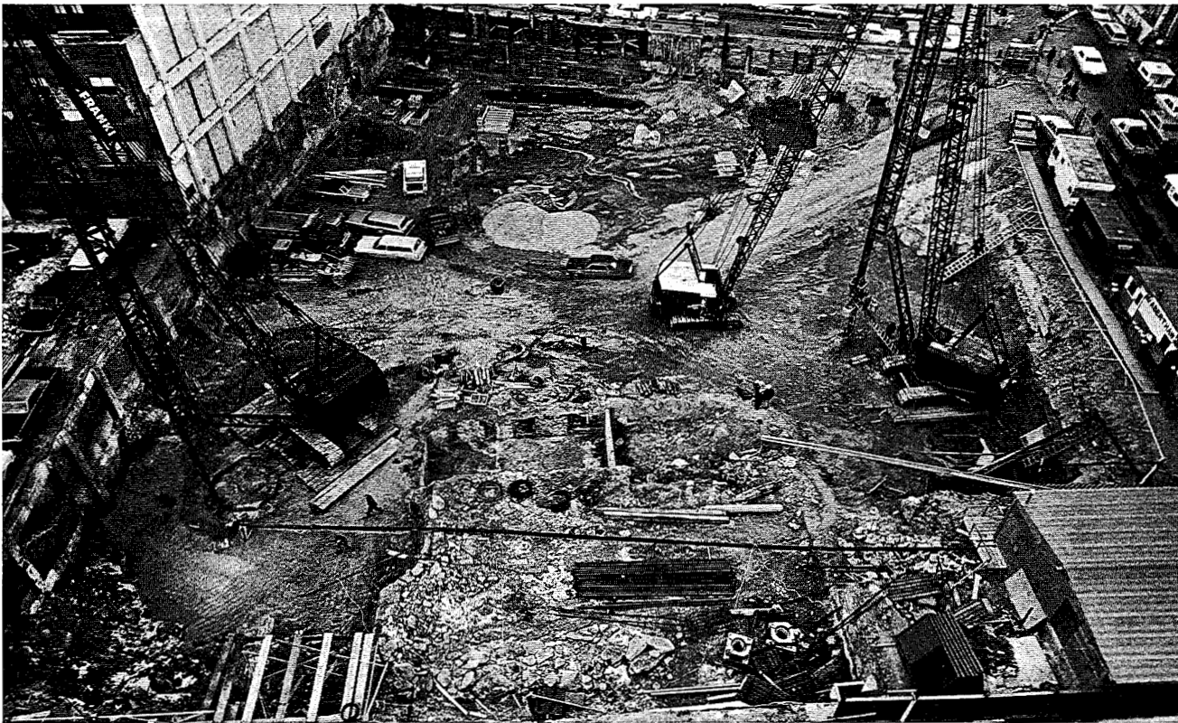
General Excavation to Basement Level; Construction of Slurry Walls for NE and SE Corner Piers in Progress (Jan. 1868)
