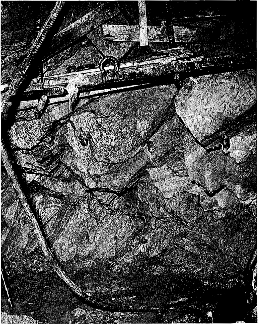
Typical Condition of Rock Undercut in Enlarged base of Pier
