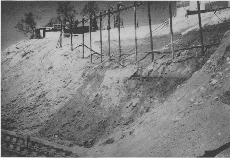
FIG. 14. ROW OF CATHODES PARTIALLY EXPOSED BY EXCAVATION OF STEEP SLOPE IN STABILIZED RIVERBANK, LITTLE PIC RIVER BRIDGE
